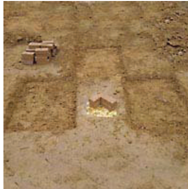
STEP 2: Cut out and remove all loose dirt from the high stress area surrounding the batter's box to a depth of 3".
