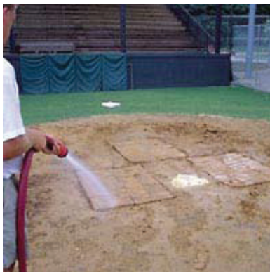
STEP 4: Once the bricks have been placed, water the cut area. Tamp the bricks into place.
