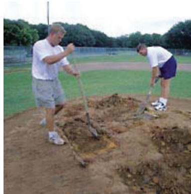
STEP 2: Cut out and remove all loose dirt from the high stress area surrounding the pitcher's mound to a depth of 3".
